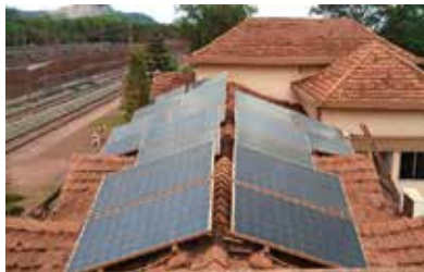
Solar Rooftop plants at Nayagarh Railway station
