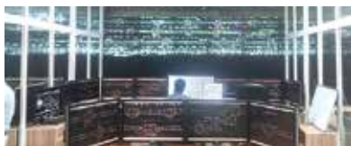
Centerlised Traffic Control System of Tundla, NCR
