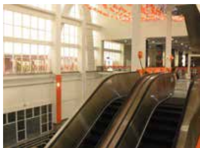
Escalator Service for Passengers at Stations
