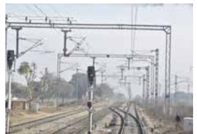
Signalling system, NWR
