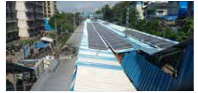
Rooftop Solar Plant
