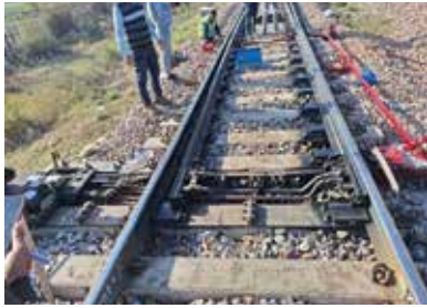
Development of 2ND drives TWS with existing Electric Point Machine
