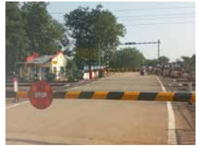
Hydraulic Railway Lifting Level Crossing Gate
