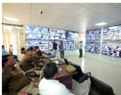
CCTV Monitoring to provide security & facilitation by team RPF.
