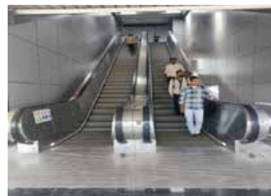
Escalator at Railway Stations for Passengers
